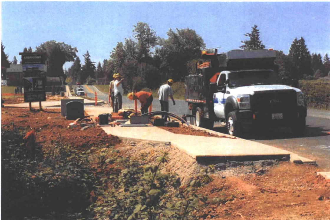
Looking south at the southwest corner of the Gustafson property. Sidewalk and electrical improvements are being made at the Urban Oaks subdivision immediately south of the subject property. Photo taken May 2015.
